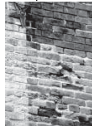
Deteriorated brick can not only be unattractive, it can be an indicator of structural problems and should be repaired as soon as possible
