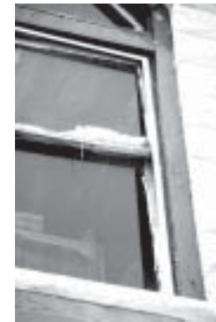
Window needing reglazing to maintain weather protection
