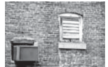
Wall "cutouts" are not only unattractive, but can also lead to significant weather related damage
